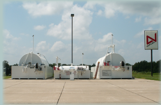
Fuel Farm- 22,500 Gal. Storage Capacity
